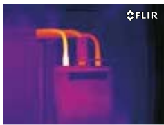
Poor connection and internal damage
